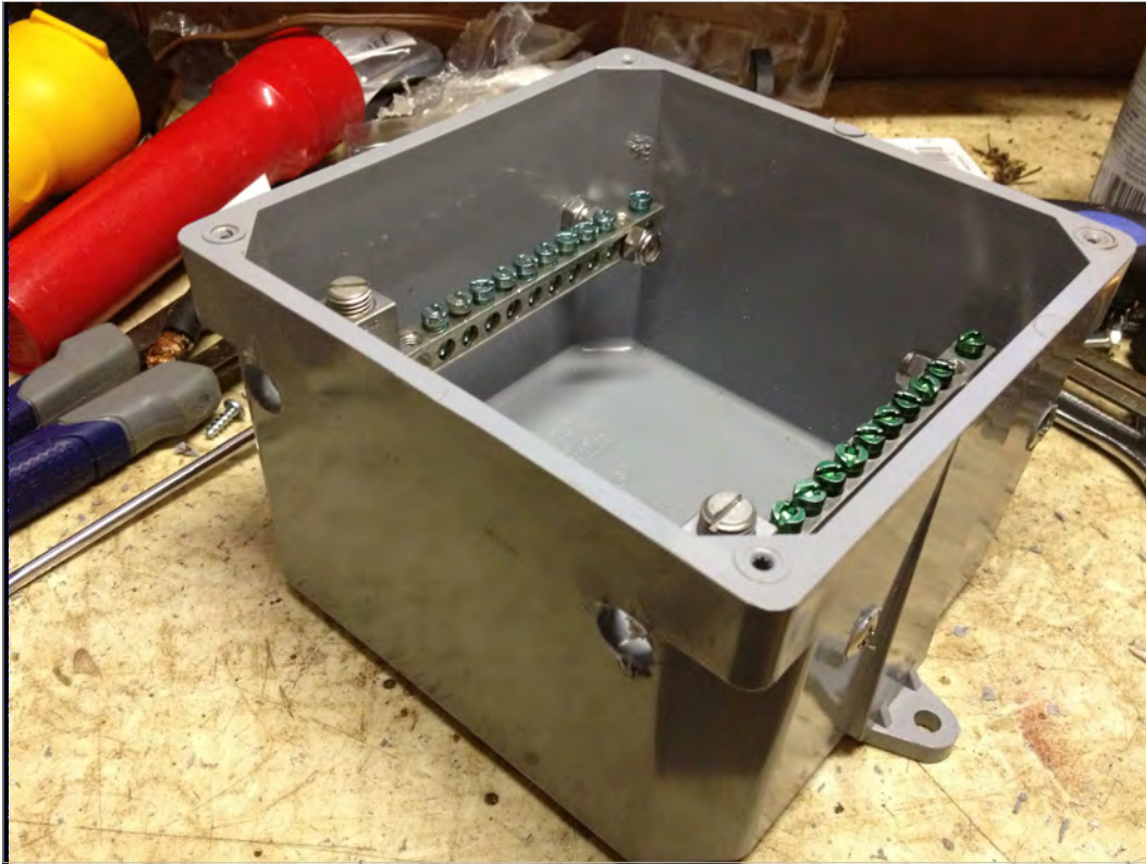
This is just another view of the PVC enclosure used to terminate each #2 cable from the battery.
